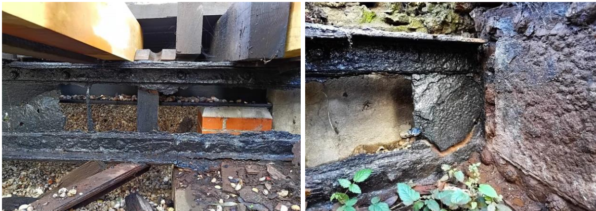
Above left: New beam behind original beam, Above Right: Old beam has risen very slightly upwards towards its original position following transfer of load to new beam (Photos: John Greenwood)
