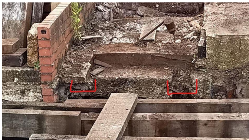
It appears the initial tracks were laid in 1922 without sleepers (John Greenwood)
